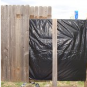
We added black tarp to prevent unwanted critters from building nests inside of the frame.
